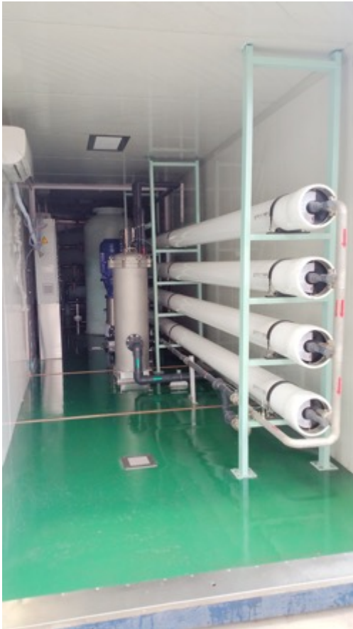
Containerlized RO - Inside
