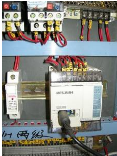
Mitsubishi PLC control system
