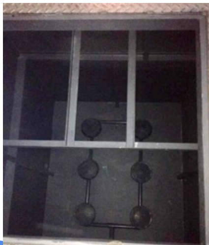
Sewage aeration device
