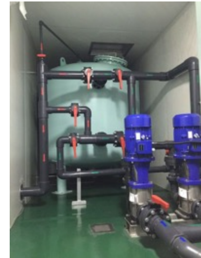
Pretreatment system & pump sets
