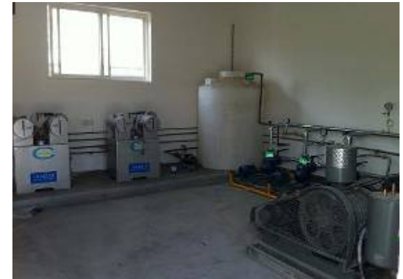
Chlorine dioxide generator sets
