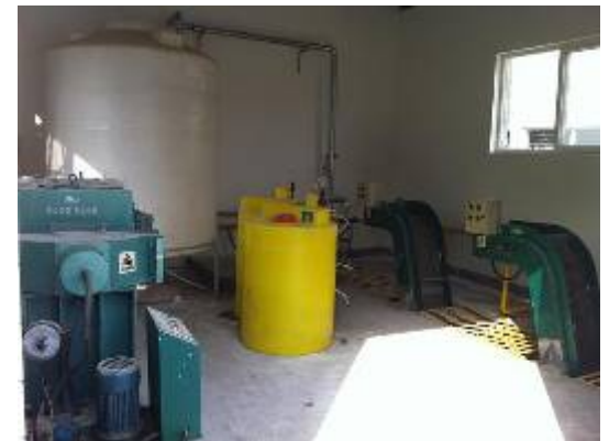
Grilling, Chemical dosing, Filter press
