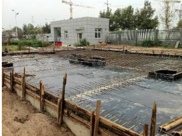
Underground treatment tank
