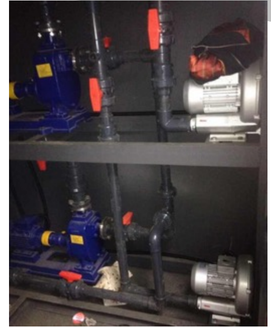
Blower and self-priming pump sets
