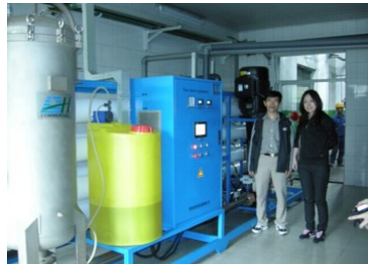
Vietnam client visiting our equipment at Pubai power plant
