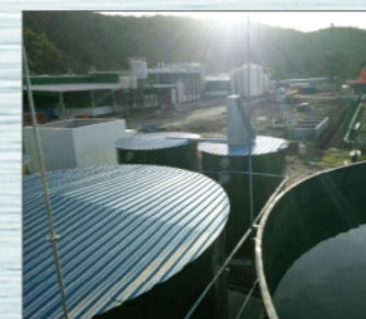
Industrial water supply
