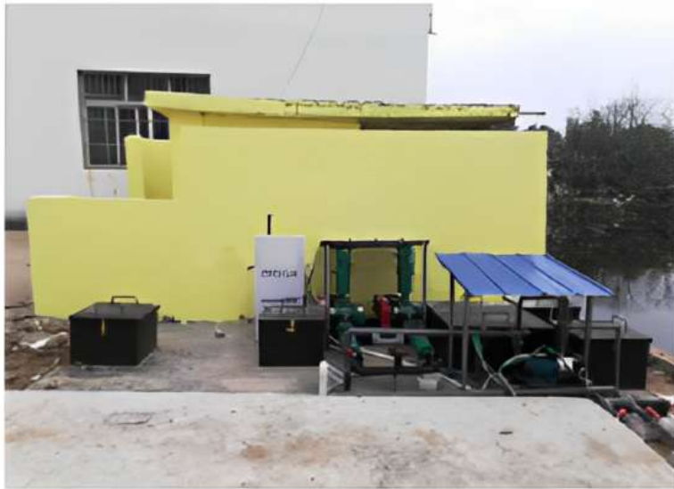
APS 50 tons/day Sewage treatment plant with air blower, water pump, sterillzer device Underground installation
