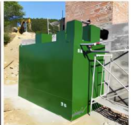
Treated water output pipeline & Air blower aeration pipeline
