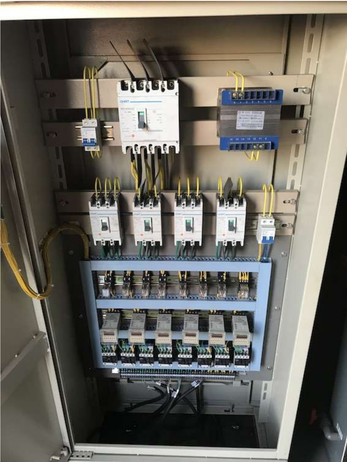
Control Cabinet ( Inside)
