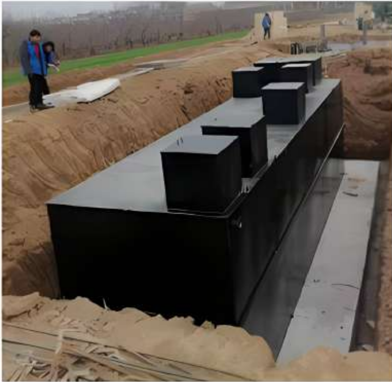
APS 80 tons/day Sewage treatment plant Underground Installation
