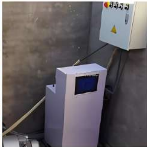
Blower & Sterilizer device & Cabinet In control room
