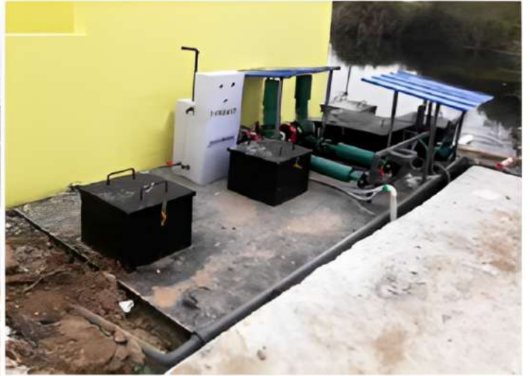
APS 50 tons/day Sewage treatment plant with air blower, water pump, sterillzer device Underground installation
