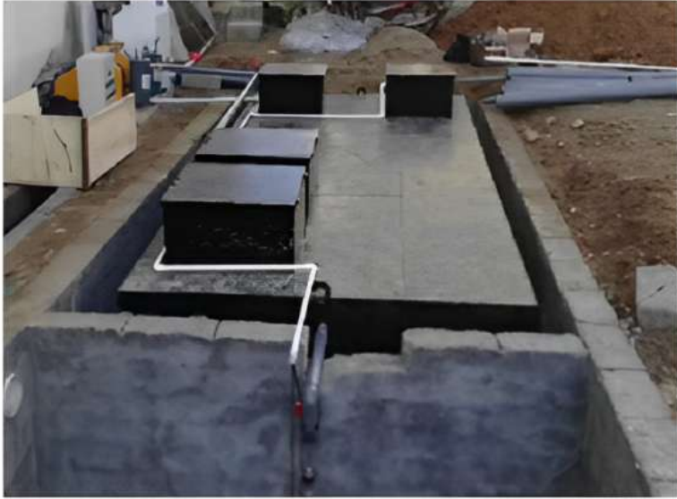
APS 40 tons/day Sewage treatment plant Underground installation
