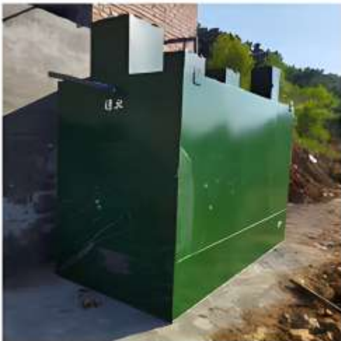
APS Equipment on ground Installation Sewage input from this side
