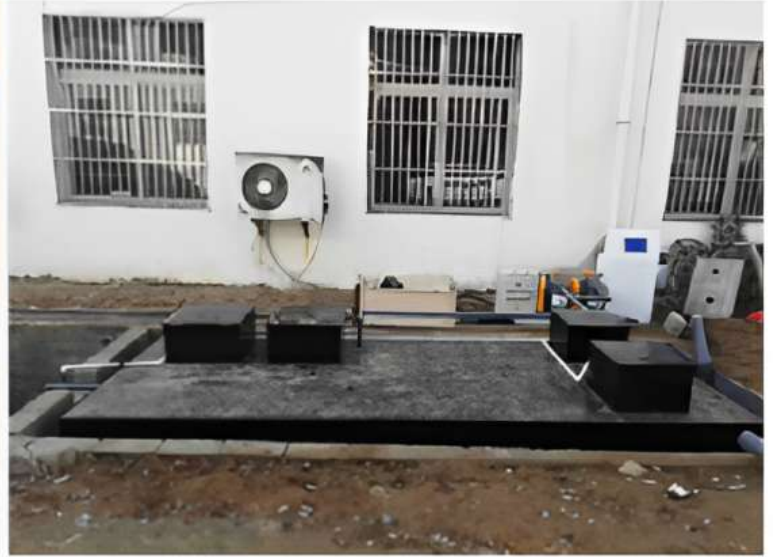
APS 40 tons/day Sewage treatment plant Underground installation
