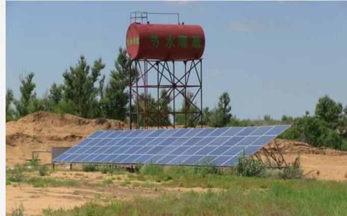
Solar pump system installed (2009)
