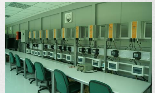
Master Control Room
