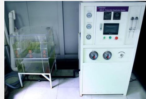
Solar Seawater/Brackish Water Desalination System Operational Testing & Data Collection
