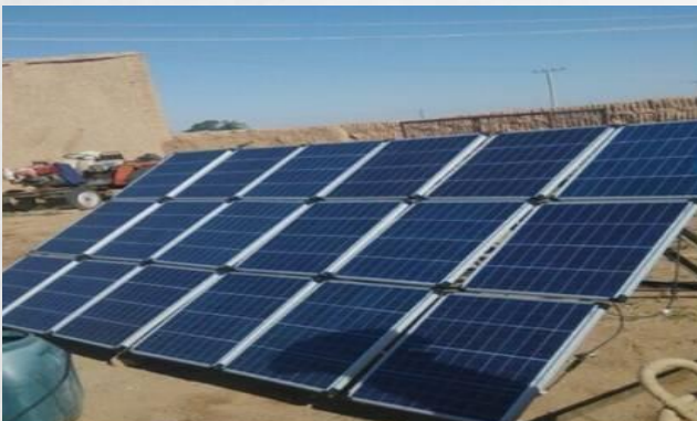
Solar pump system
