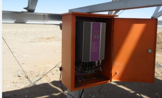
Soalr Pumping Inverter
