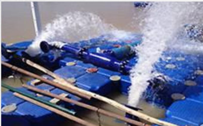
Heavy water flow
