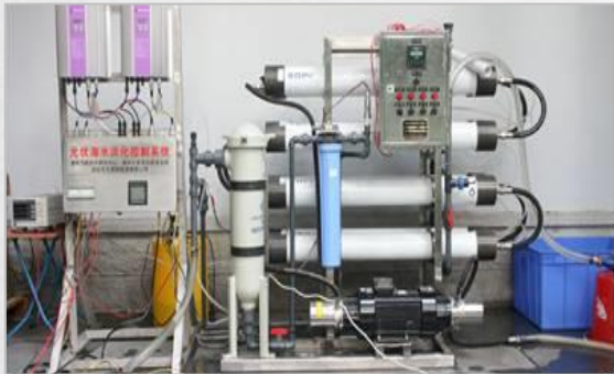
Master control equipments
