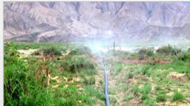
Spray irrigation system
