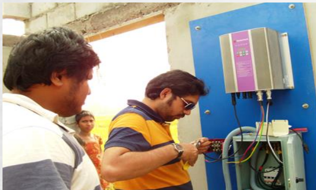
Solar pumping inverter installed
