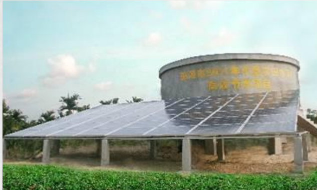
Solar pump system
