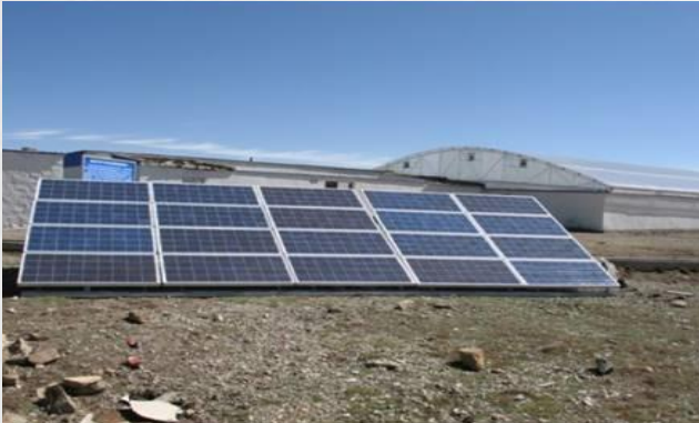
Solar pump system
