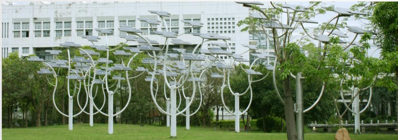
Solar Tree Operational Testing & Data Collection
