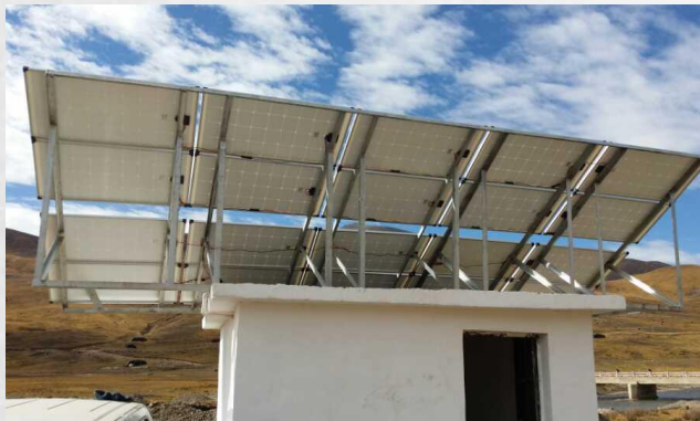
Solar Array and Control Room
